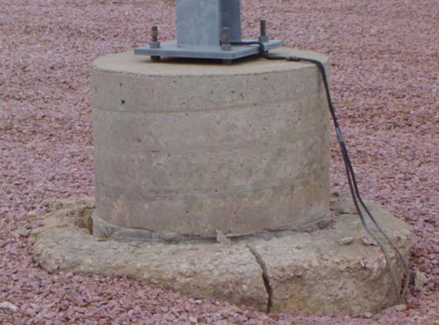
If a 30" diameter pier x 8'-0" into the ground still heaves, what can we do?
