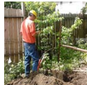
GPS new underground secondary line
